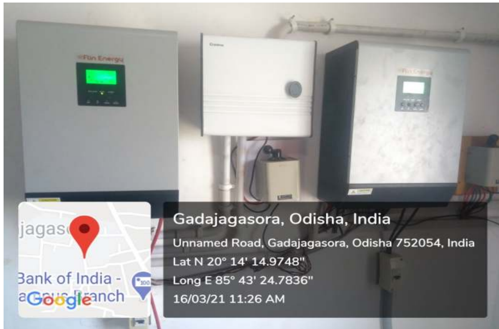
(Solar Panel Inverter Switch)
