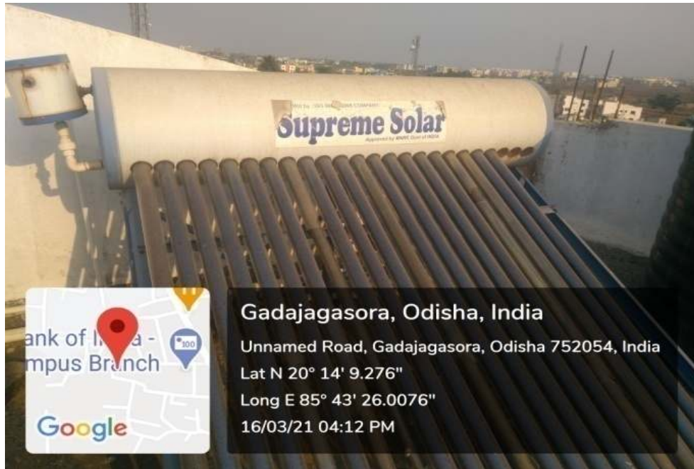
(Solar Water Heater placed in Roof top of Central Mess)
