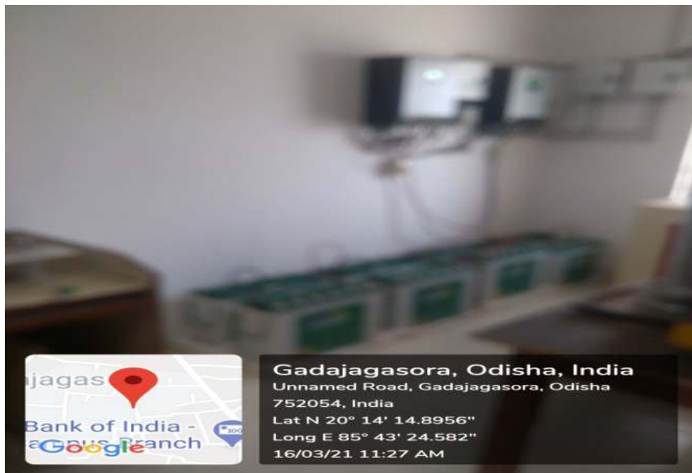
(Solar Panel Inverter with Battery)
