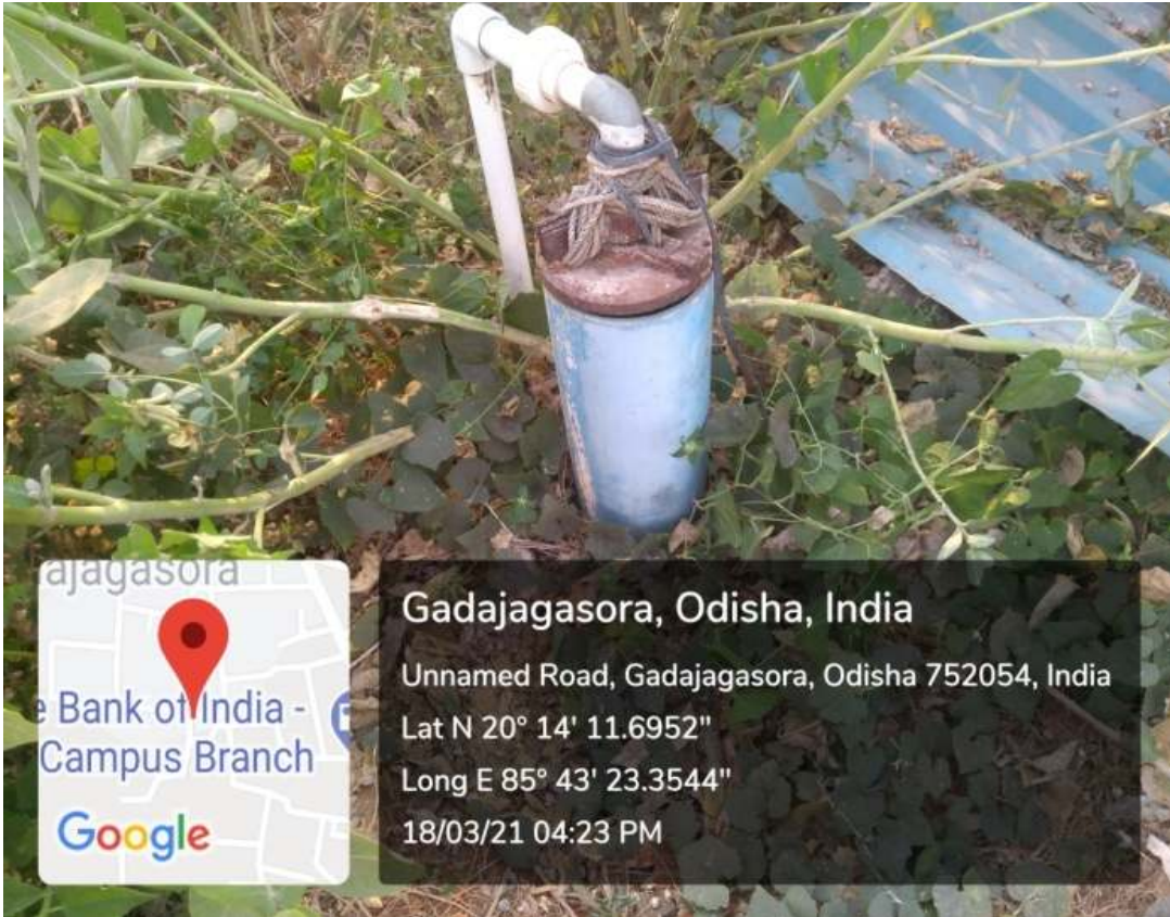
(Bore Well No-4)
