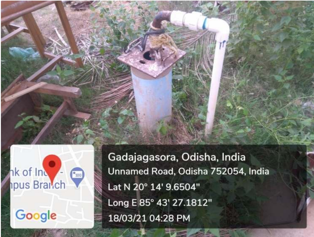
(Bore Well No-8)
