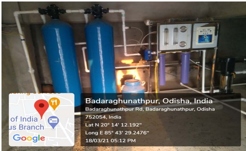
(1000 liter RO Facility for Drinking Water)
