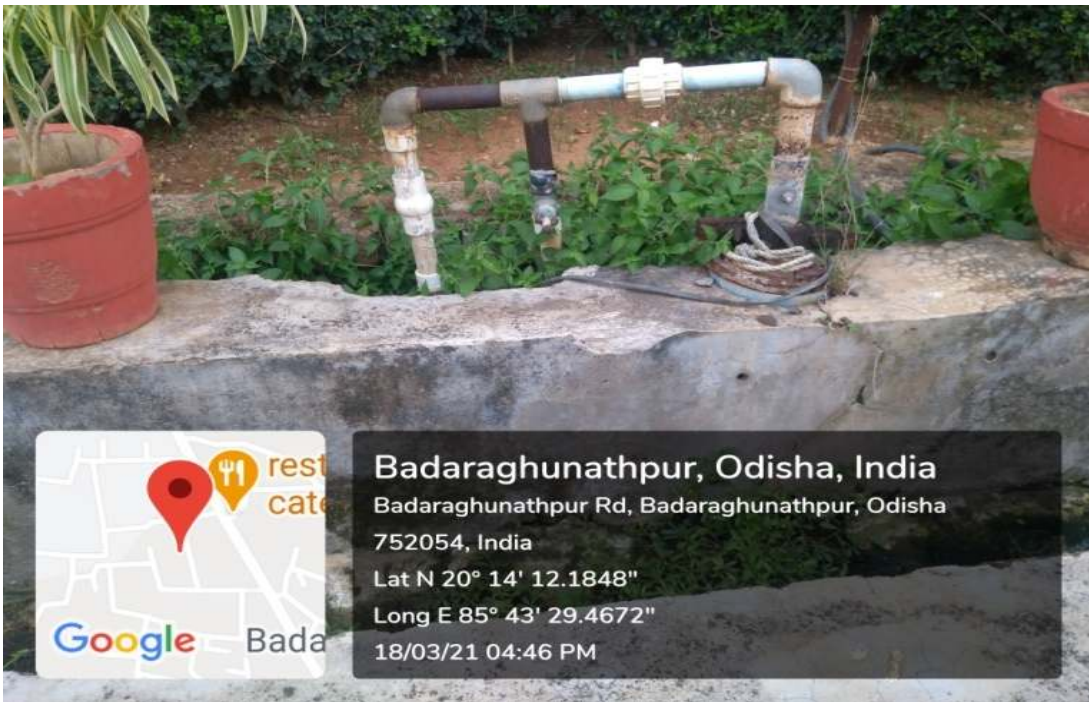
(Bore Well No-1)
