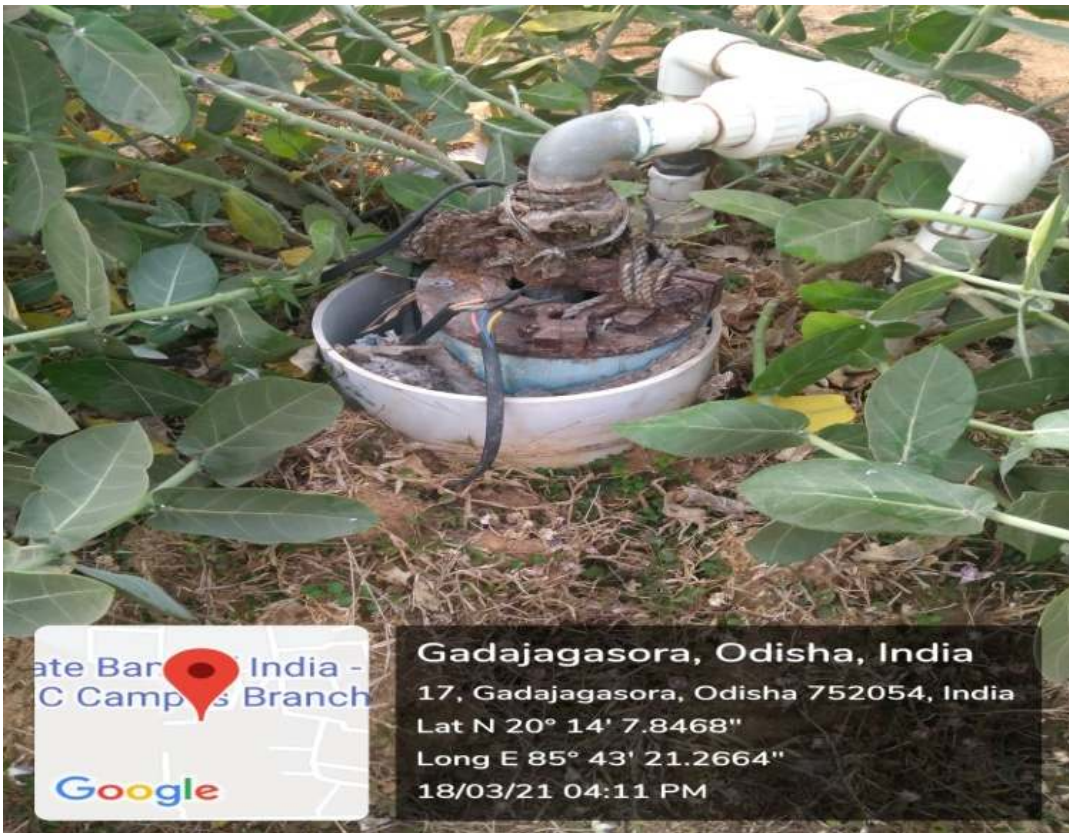
(Bore Well No-3)
