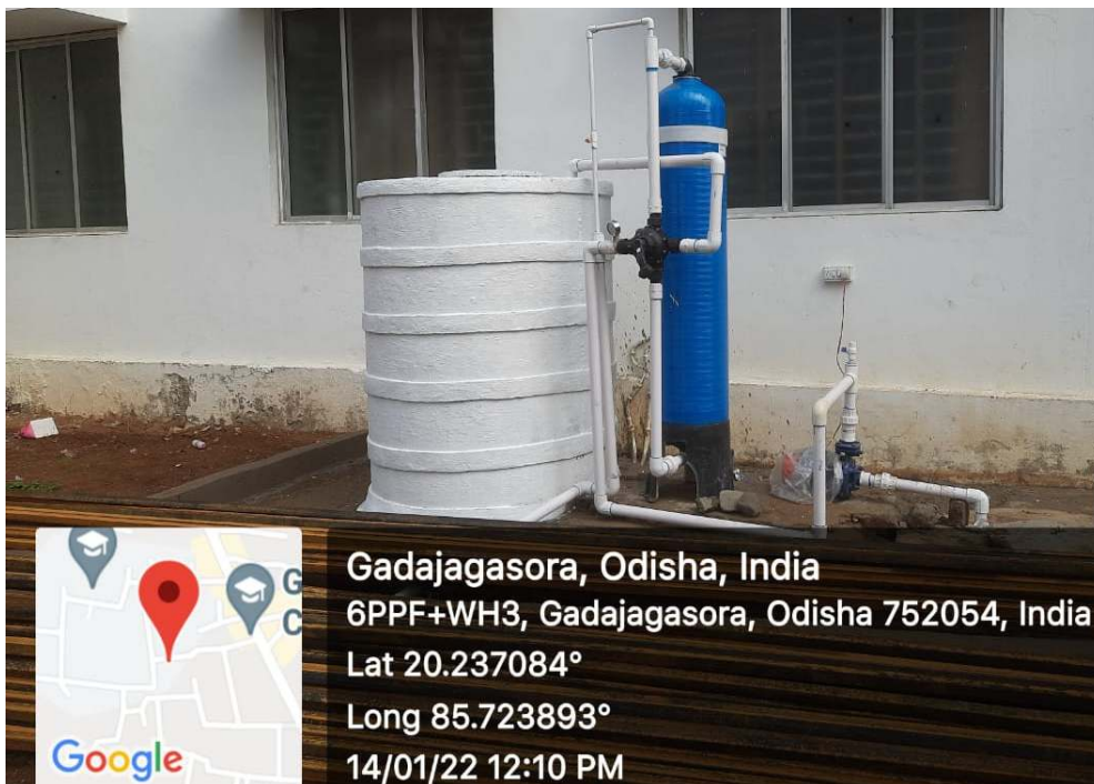
(Rain Water harvesting)
