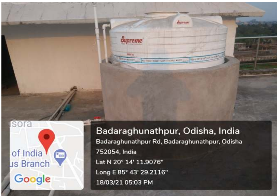
(Water Tank at the roof top in Academic Block)
