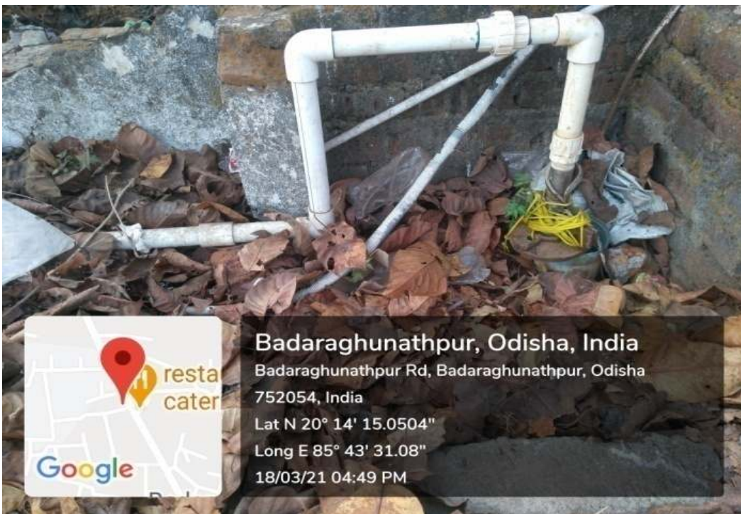
(Bore Well No-5)
