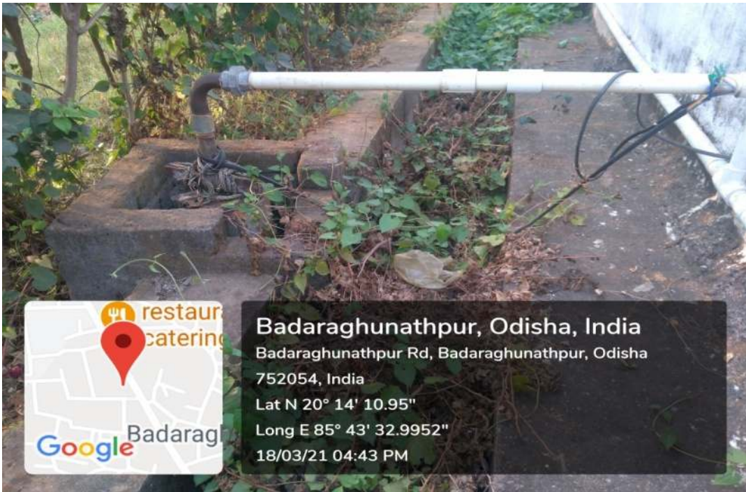
(Bore Well No-2)
