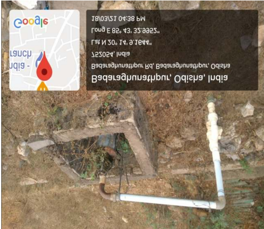
(Bore Well No-6)
